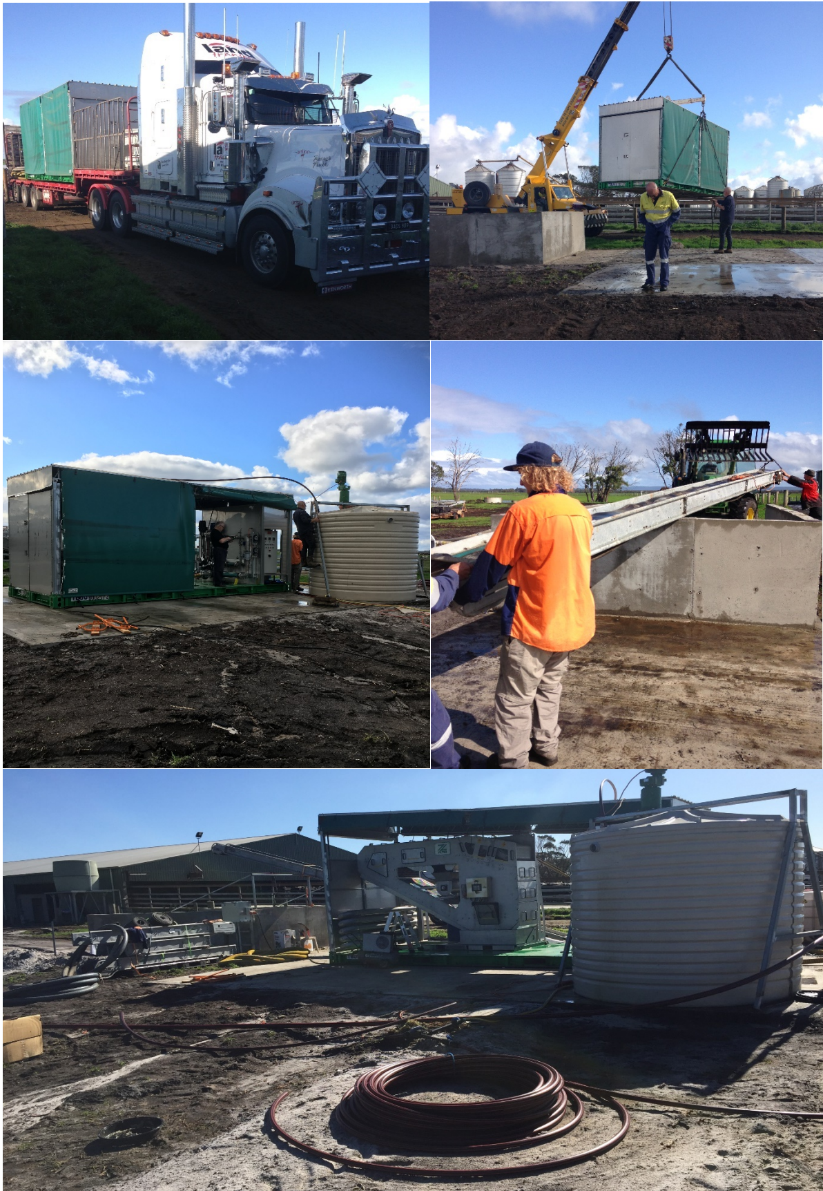
Figure 4 Skid-mounted Z-filter unit and ancillaries upon delivery and during installation at the dairy trial site
