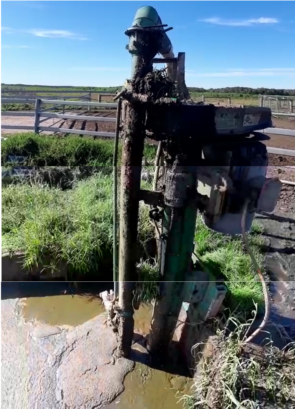
Figure 13 Large existing effluent transfer pump, which was repurposed for recirculation mixing of the Z-Filter.
